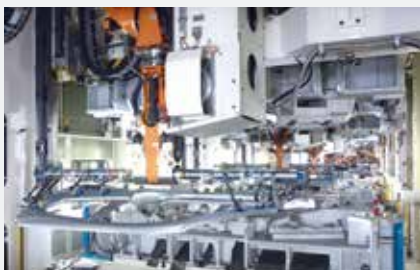
Crossbar Feeder Automation.
