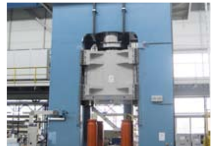
Trimming and calibrating press with a press force of 2,000 metric tons (2,250 US tons)
